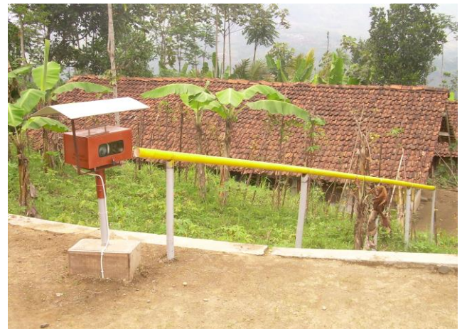
Figure 1 Automatic extensometer installed at the upper slope at a densely populated area.
