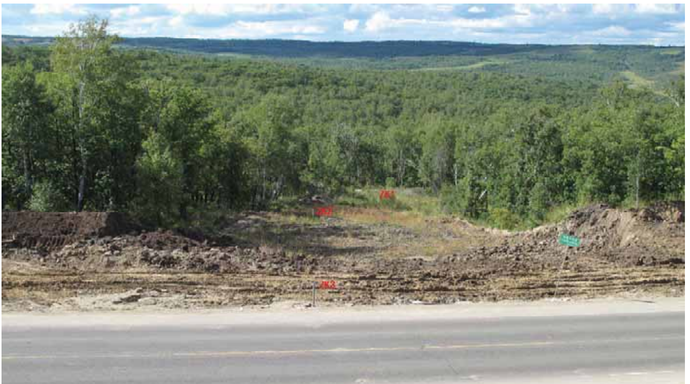
Figure 2 K178+530 landslide photo
