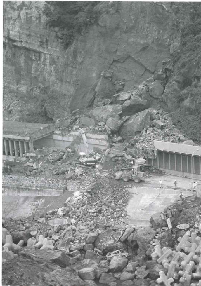
Fig. 2 The rockfall in Echizen-cho (by courtesy of the Yomiuri Shinbun).
