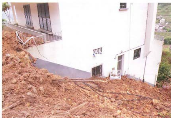
Fig. 5 A house destroyed by the earthflow.
