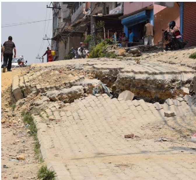
Figure 4 Main scarp of the landslide.
