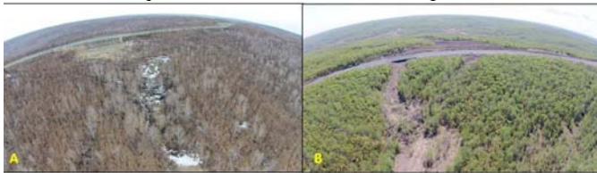
Figure 7: anti-slide piles to reinforce(K177+550) and building bridge to take place the road(K178+530) to reach a solid foundation for support
