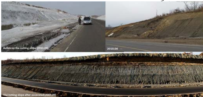
Figure 4: In digging section: icing in winter and slope slump in spring
