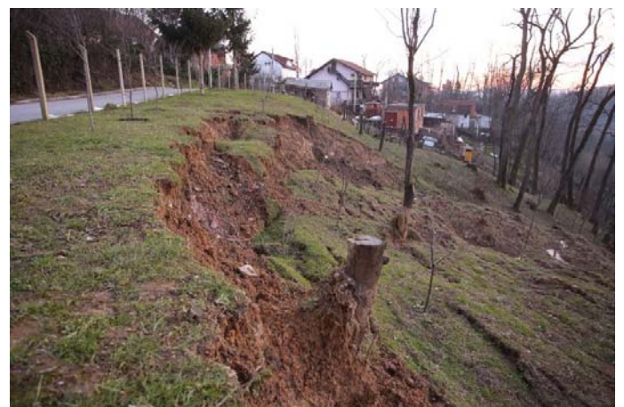
Figure 2 Typical soil slide developed in Plio-Quaternary soils in the City of Zagreb. The cause was concentrated flow of superficial water from road which activated sliding during heavy precipitation in 2013 (Bernat Gazibara et al. 2017b)
