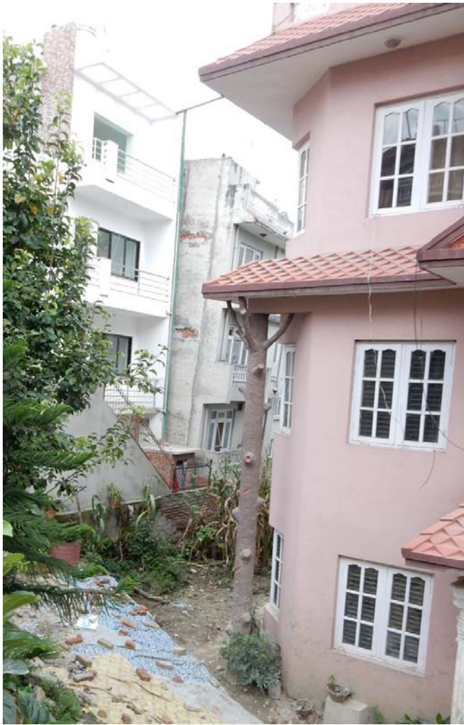
Figure 3 Distressed building due to the landslide.
