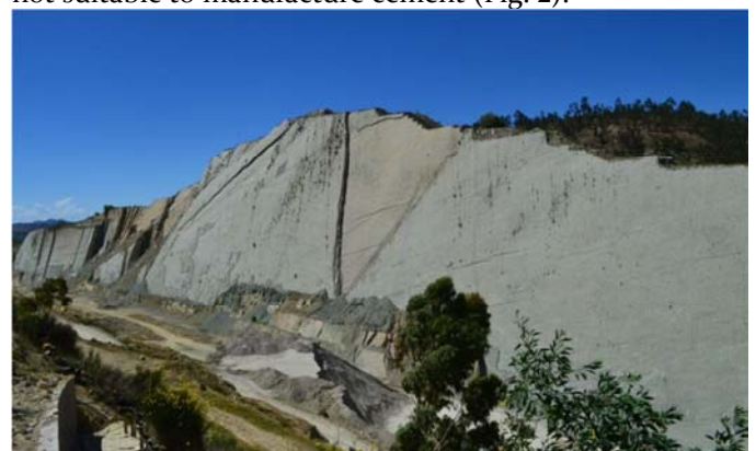
Figure 2 A partial view of Calorcko paleoichnic cliff. In the middle, the so called "advanced deterioration triangle" collapsed in February 2010.
