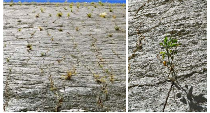
Figure 7 Plants growing into the cracks
