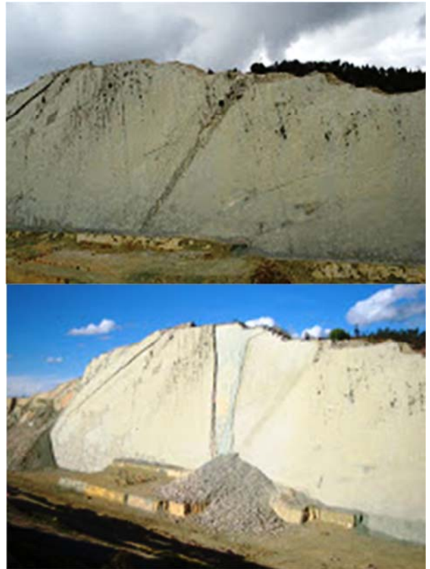
Figure 4 The paleoichnic cliff before and immediately after the February 2010 dip slope failure (Pictures: Willy Jordán)
