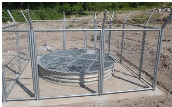
Fig. 4 Drainage well from the outside, with its protection cover and surrounding fence to avoid intruders. (Taken by Froilán Castro, 2013)
