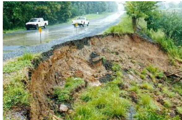
Fig. 1 Rotational slip in the Panamerican Highway, Tole, Chiriqui province (photo taken by Ministry of Public Work, Panamá in 2001)
