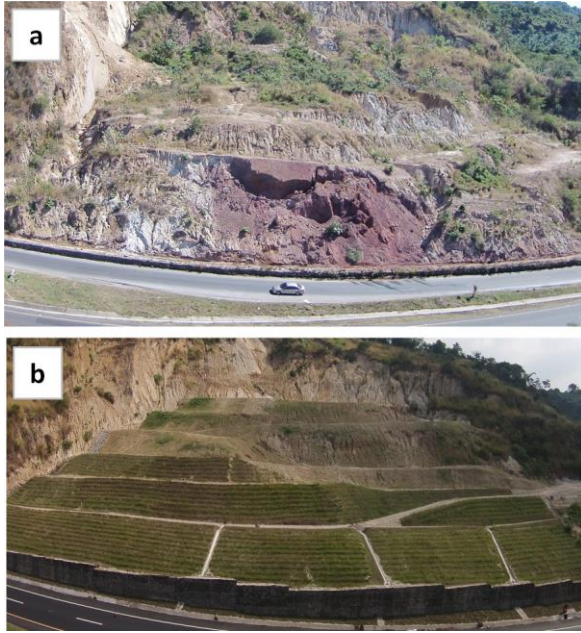
Fig. 6 a. Landslide located at the km 18.5 of the CA-01 East route in El Salvador. It occurred during the night of January 17 th , 2009 (photograph taken by Yuri Rodriguez on January 5 th , 2014). b. Control measure applied to the affected slope (photograph taken by Jorge Urrutia on December 17 th , 2015)
