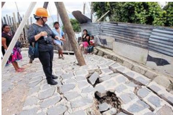
Fig.3 Location of a damage level 4 (see Fig. 2), presenting the structural damage of the road (Photography by Xiomara Robleda, 2013).
