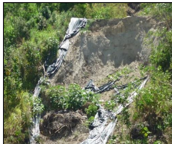
Fig. 2 Landslide in San Francisco Street, Antiguo Cuscatlán, El Salvador, which occurred during an unspecified rainfall event in October 2010 (photograph taken by Alonso Alfaro on March 18 th , 2011)
