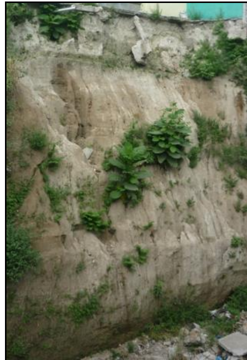
Fig. 4 Erosion problem in the Tierra Blanca formation of the Jardines del Pepeto 3 community, Soyapango, El Salvador. It occurred during the passage of Hurricane Ida in 2009 (photograph taken by Aleyda Montoya on May 25 th , 2011)
