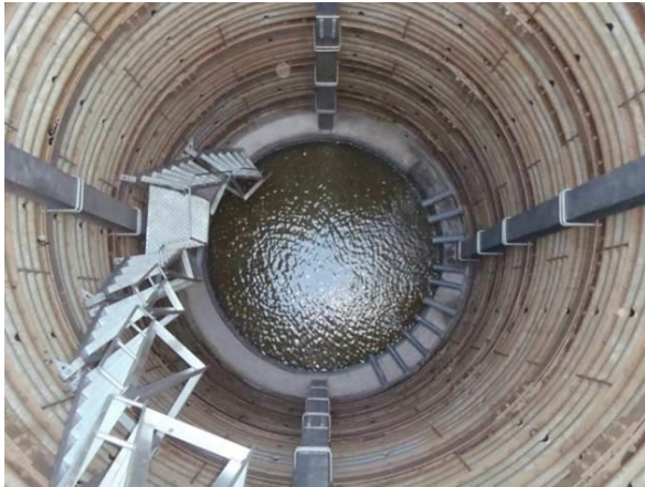
Fig. 5 Drainage well seen from above with its ladder for maintenance and at the bottom water is captured from the intake pipes. (Taken by Froilán Castro, 2013)
