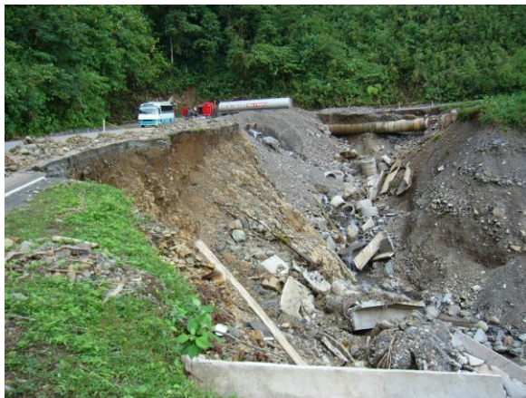
Fig. 2 Road slip at Chiriqui-Bocas del Toro conditioned by the presence of geological faults and poor design of drainage system (photo taken by Eric Chichaco in 2012)
