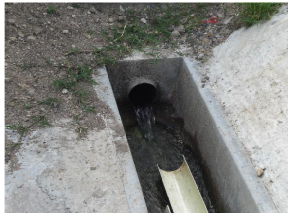
Fig. 9 Drainage pipe from well No.2 in Reparto connected to the canal to finally discharge to the residual waters canal in this area. (Taken by Froilán Castro, 2013).
