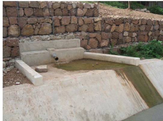
Fig. 8 Drainage pipe from well No.6 in Berrinche connected to the canal to finally discharge to the river. (Taken by Froilán Castro, 2013)
