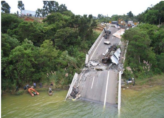
Figure 1 Bridge fall over the Capivari River caused by landslides, affecting the most important Brazilian highway that connects the southeastern and southern regions (2005).
