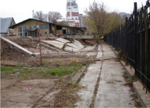
Figure 4. Wall disruption of sliding sub block and the widest part of slipping down the under rim part at the territory of Holy Trinity temple (12.10.06), sliding area Choroshevo-1
