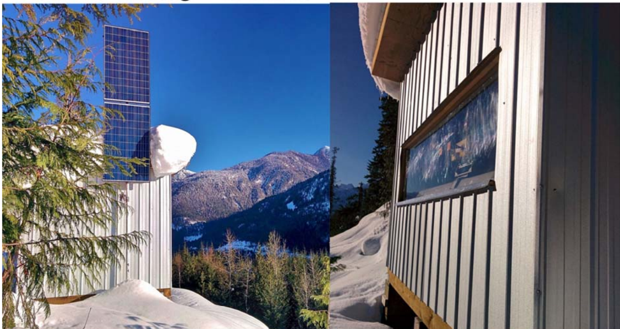
Fig 6. GB-InSAR installation up stream of the BCHydro's Revelstoke dam, British Columbia, Canada. Installation is monitoring the unstable slope at Checkerboard Creek. Note: location is remote without power supply, steep north-south valley, and some of the highest amounts of snow accumulation in Canada.
